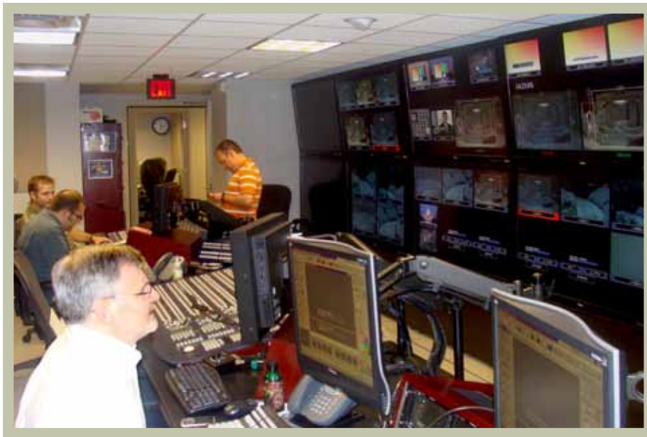
New House Recording Studio control room.
