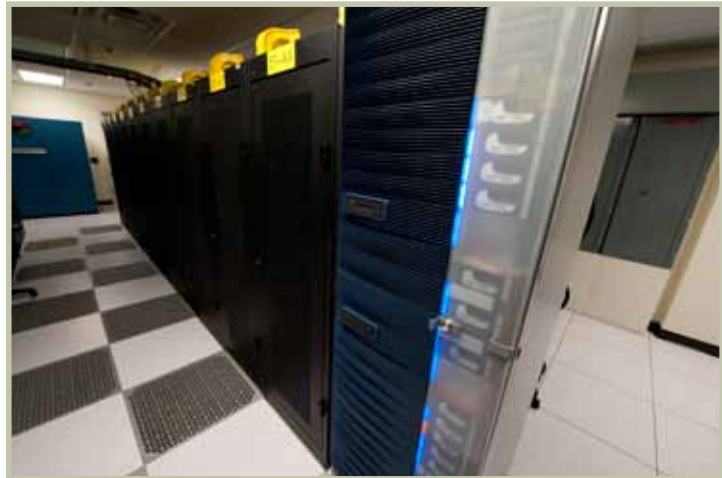
A blade frame server, right, uses far less energy than traditional servers.
